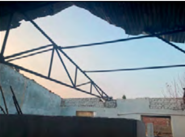
Roof tops blown off (JLM)
